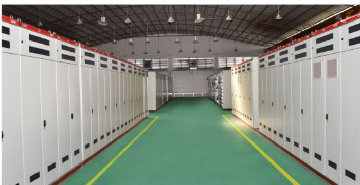
高低压柜生产车间 | High and low voltage cabinet production workshop |
