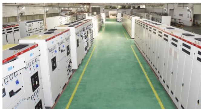
高低压柜生产车间 | High and low voltage cabinet production workshop
